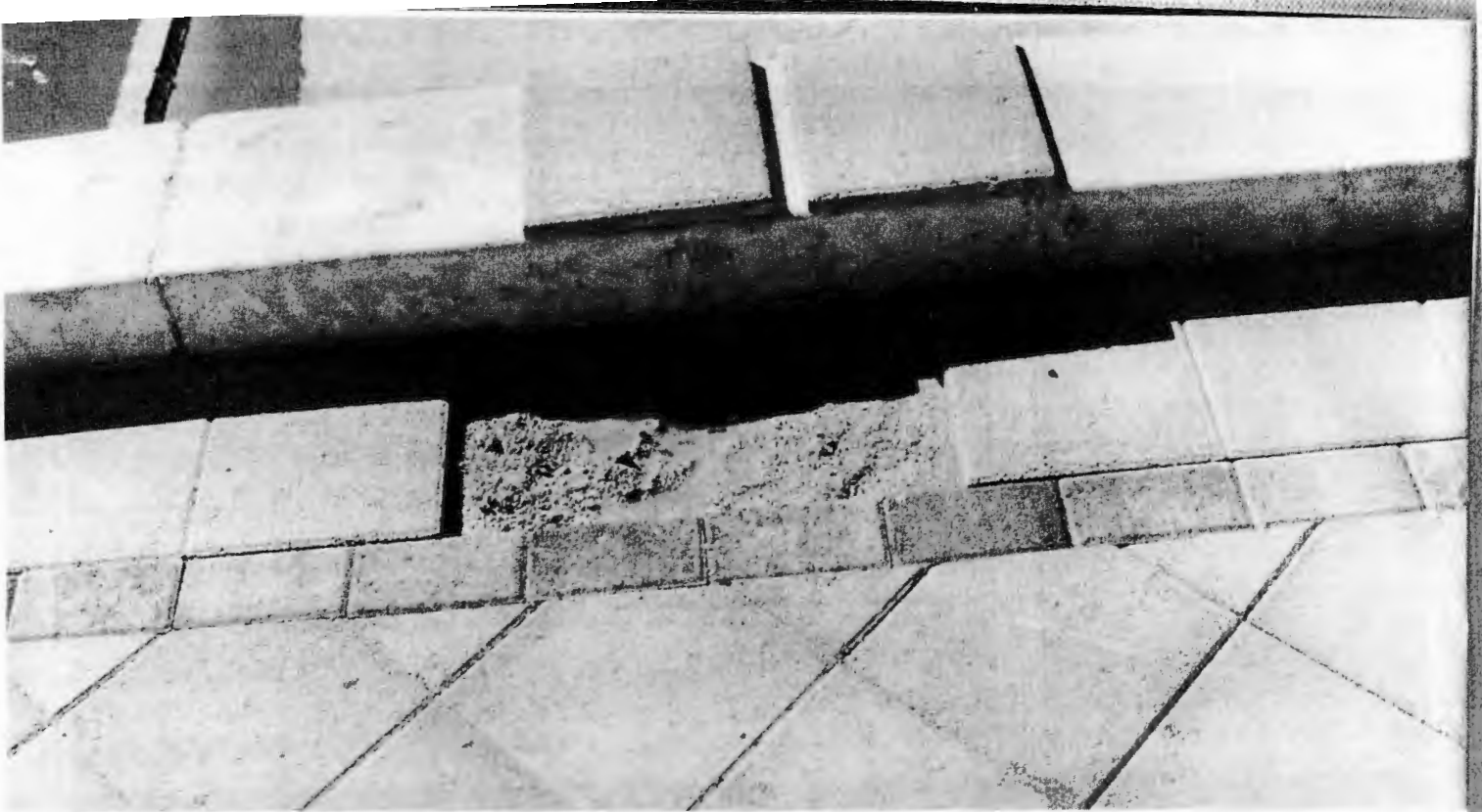
Pavers can hide areas of ponding water and water intrusion.
