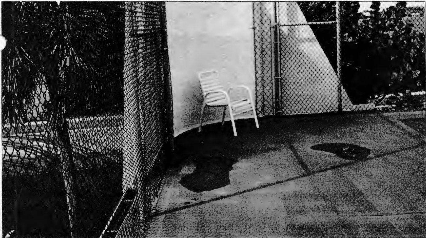
Ponding water deteriorates waterproof coatings and can cause slip hazards.
